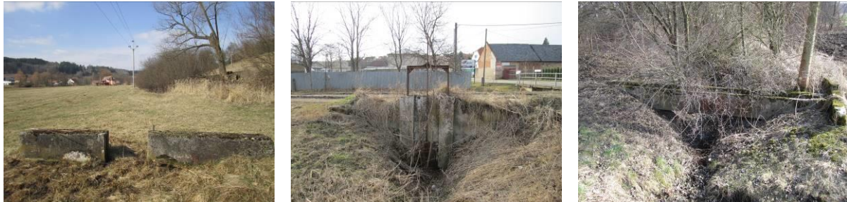
Figure 4 A setting device at none exist drive in 2017 (on the left), Example of a drain in 2017 (in the middle), An aqueduct across nameless watercourse in 2017 (on the right)
